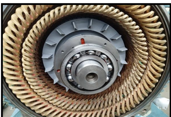
Fig. 5. NDE Bearing renewal (Isolated).
